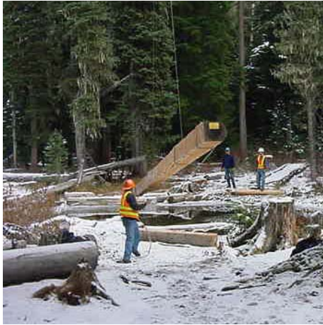
New Arch Rock Trail bridge being flown to the bridge site. November 2003
