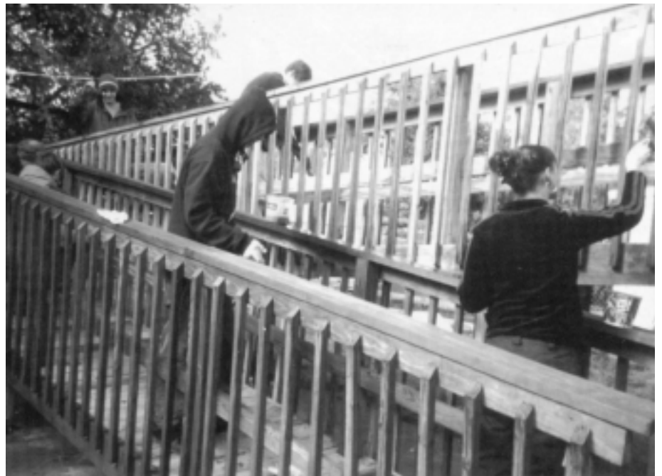
Through the Community Connections program, these East Montpelier School students worked with Chore Buddies, a program of the Vermont Center for Independent Living, to stain ramps for people with disabilities in Central Vermont. VHCB provides funds to VCIL to design and build ramps and make accessibility modifications for homes and apartments statewide.
