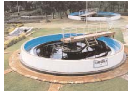
Waste water treatment plant
