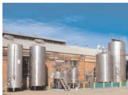
Storage tanks for recovered water
