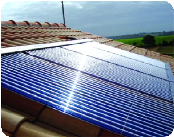
Solar Hot Water
